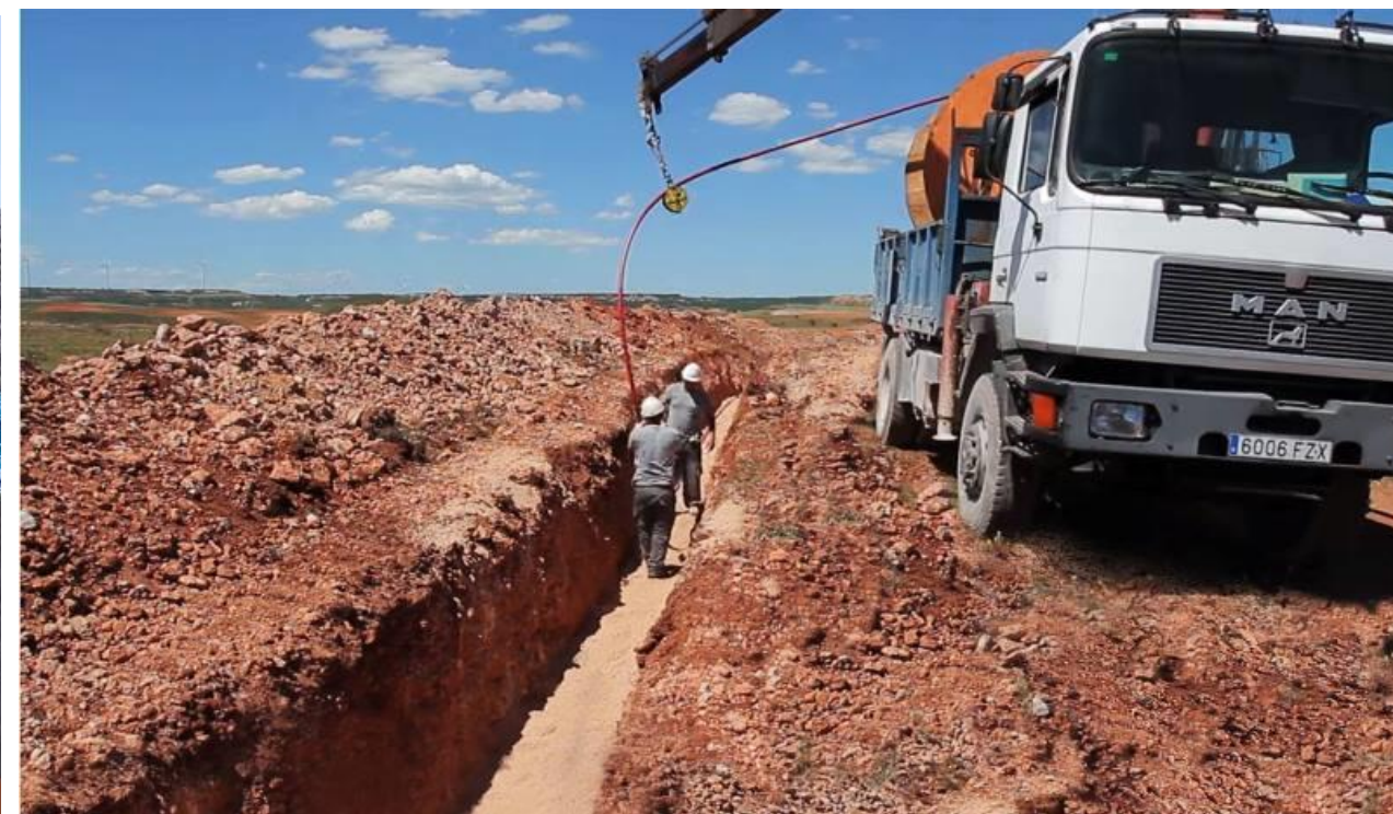
Trenches with electric cables everywhere
